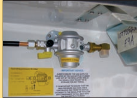
Truma Regulator already supplied with a 90 degree elbow fitted on its side close to a reinforcing strut
