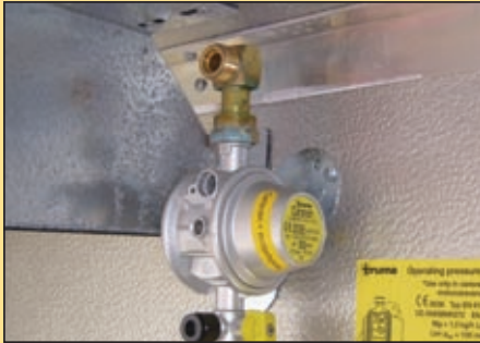
Truma Regulator already supplied with a 90 degree elbow fitted close to a reinforcing strut on the left
