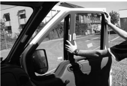
B24: Insert frame and press against door. Transfer the 6 drill holes to the door frame.
